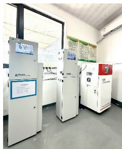
Wastewater Online Monitoring Equipment
